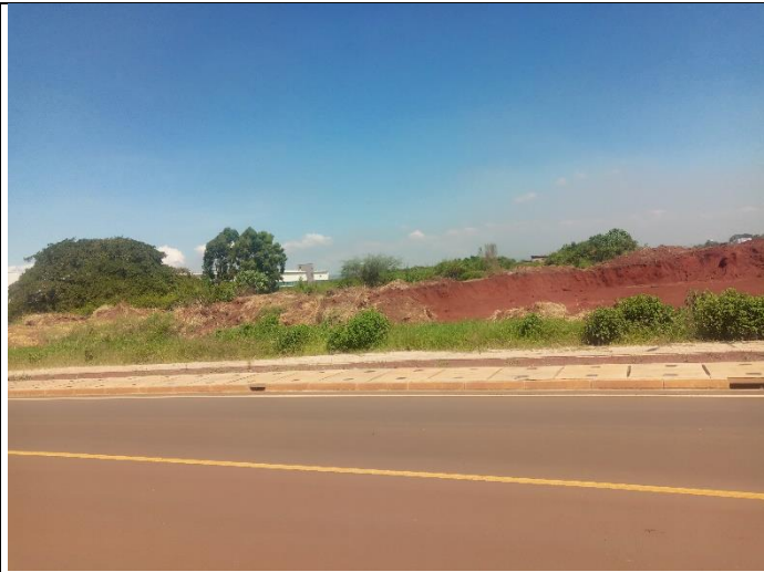
Project Site: Access road available, Mugumo tree on the left with a few eucalyptus trees behind it, levelling on-going under Tatu City.
