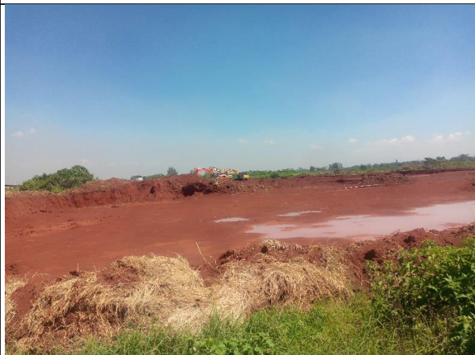
On-going grading of the Project Site by Tatu City guided by the approved ESIA Study conducted for the wider development of the Precinct 3BA in which the Project Site is located
